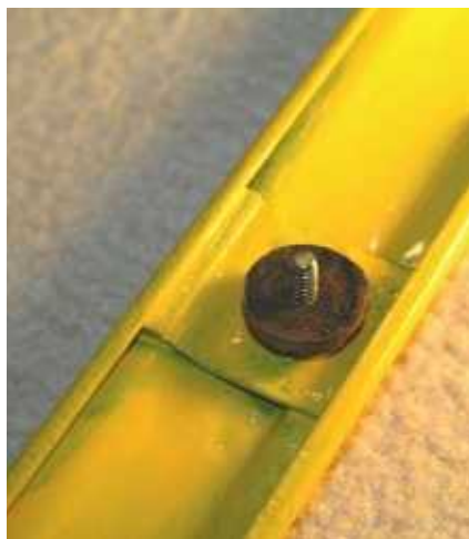
One of the six lower fixings that secure the bottom of the window frame surround to the side of the shell. Thankfully my dad, Peter, came to the rescue and cleaned the delicate threads up as using a wire brush would have been too harsh on them.
